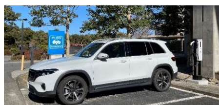
EV charging Station
